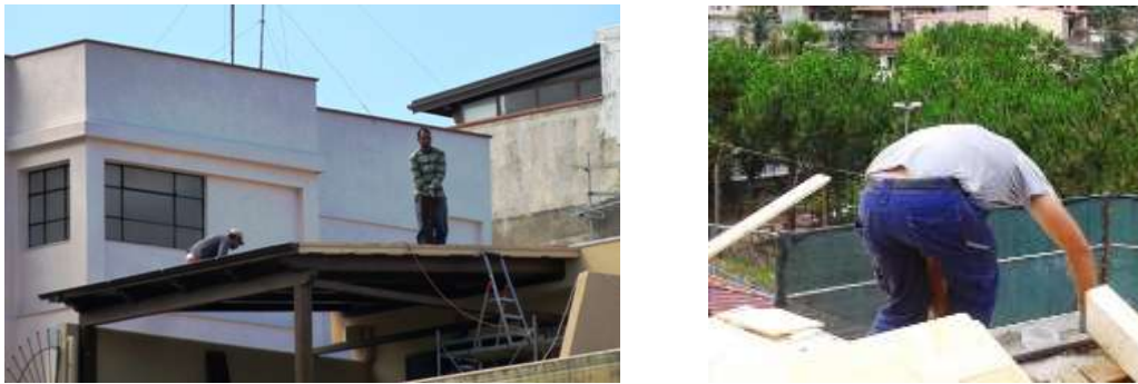
Figure 1. Workers performing maintenance coverage without necessary protection.
