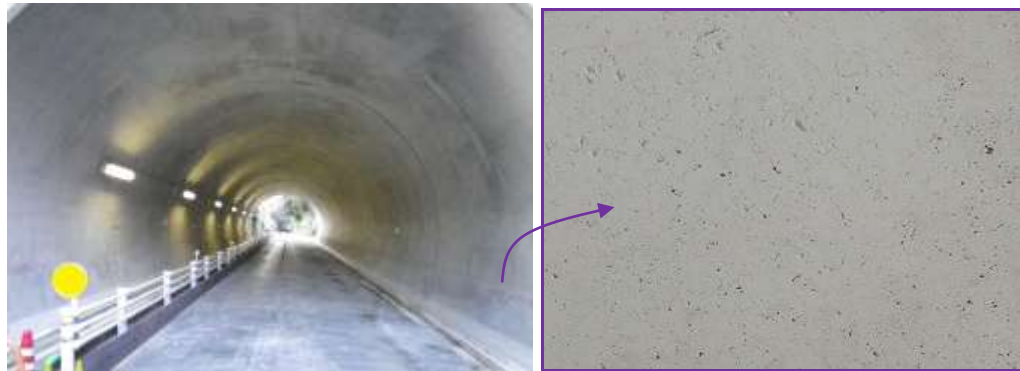
Figure 1. Bubbles on the side wall of a tunnel lining.
