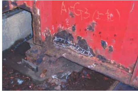
Figure 2. Peeling conditions between webs and lower flanges near supports.
