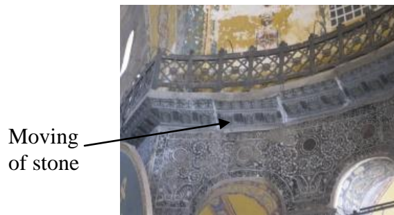
Figure 6. Problems at the south west second cornice.
