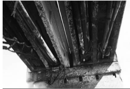
Figure 2. Damages of span five.
