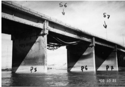
Figure 1. Damages of bridge.
