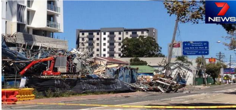
Figure 2. The collapsed scaffold at the Mascot building site.
