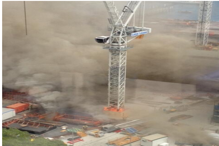
Figure 3. The crane incident at the Barangaroo development project near CBD.
