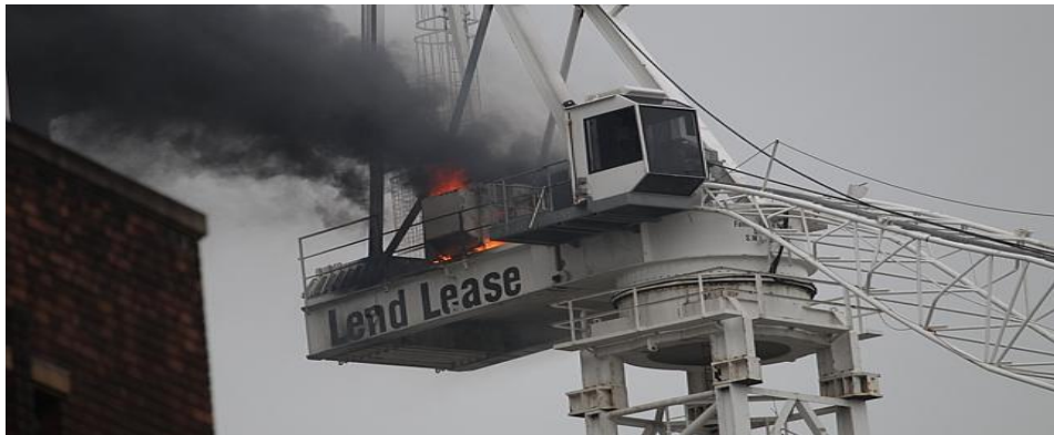
Figure 1. The tower crane at Ultimo construction site on fire.
