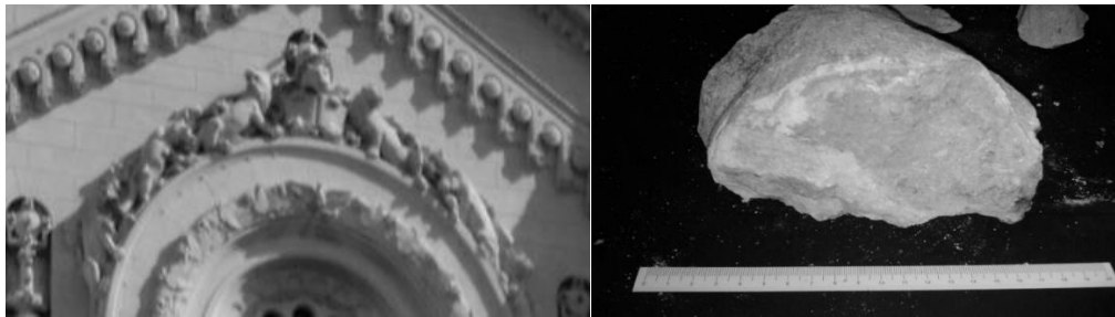
Figure 2. The large fragments that collapsed were the head of a lion decoration that overhung the rose window.
