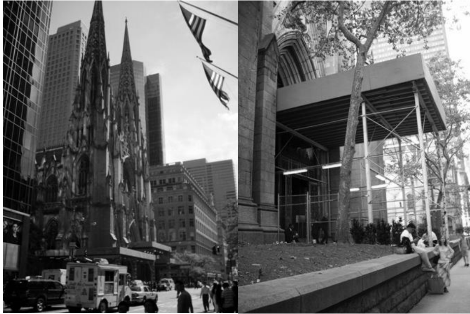
Figure 1. Works provisional after the collapses of architectural elements in the St. Patrick's Cathedral in New York (2011).
