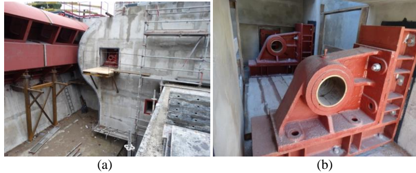
Figure 3. A view of the position of the sleeves: a) in the sluice wall, b) the mutual positioning of the sleeves (view from the inside of the sluice).
