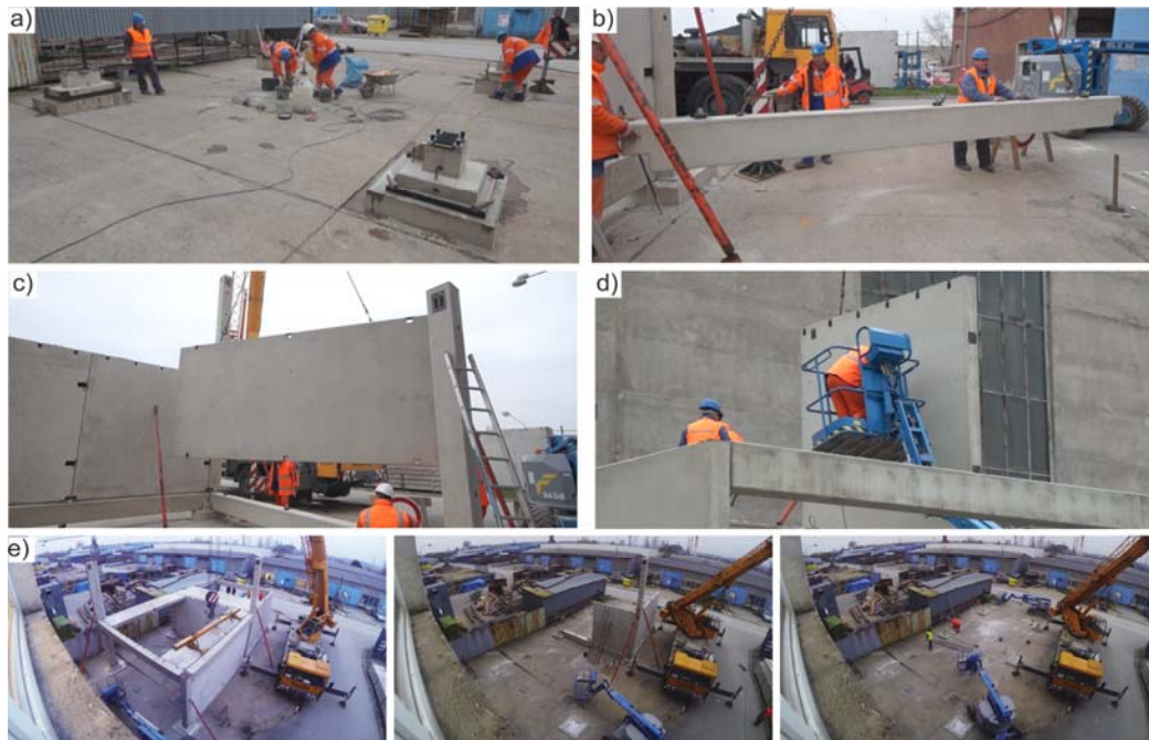
Figure 4. a) Preparation of foundations, b) Assembly of foundation beam, c) Assembly of a stiffening diaphragm (bracing wall), d) Assembly of load bearing wall in second floor, e) Gradual disassembly of the structure.
