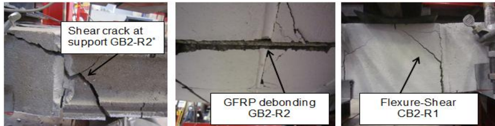
Figure 4. Observed modes of failure.
