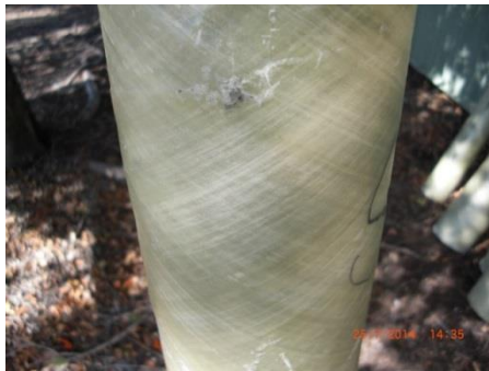
Figure 3. Change of texture of FRP column.
