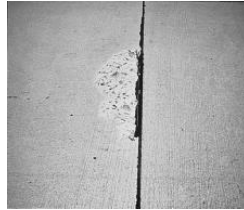
Figure 1. Beginning spall (Fowler et al. 2008).
