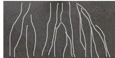
Figure 3. Typical crack pattern in ECCN0.5.
