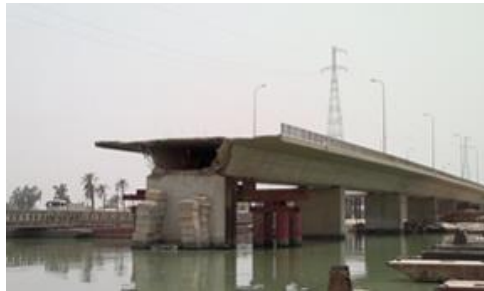
Figure 2. Damages of bridge
