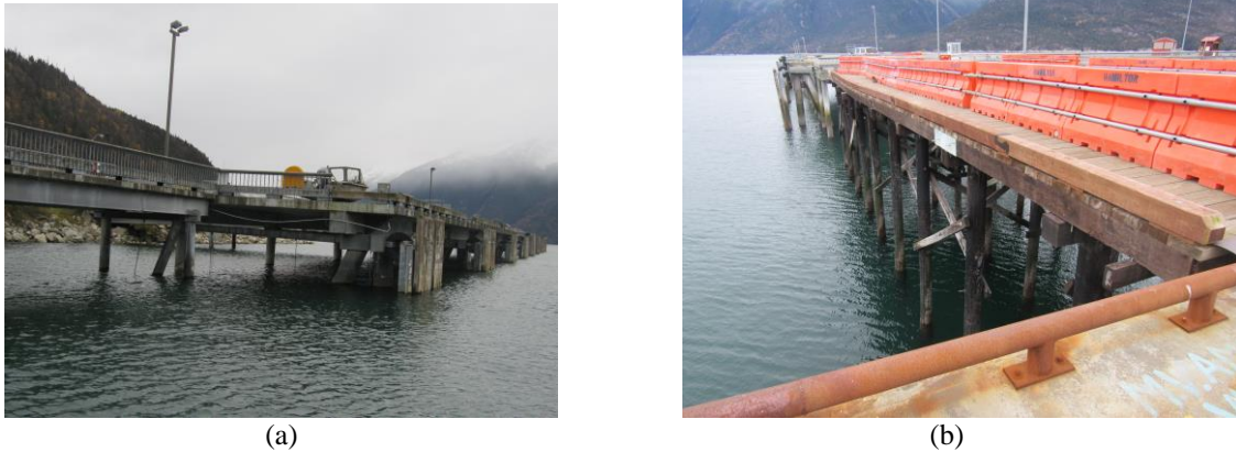
Figure 1. Piers with a) timber deck on timber piles, and b) concrete deck on steel pipe piles.
