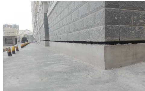
Figure 4. The crack of the tilting building
