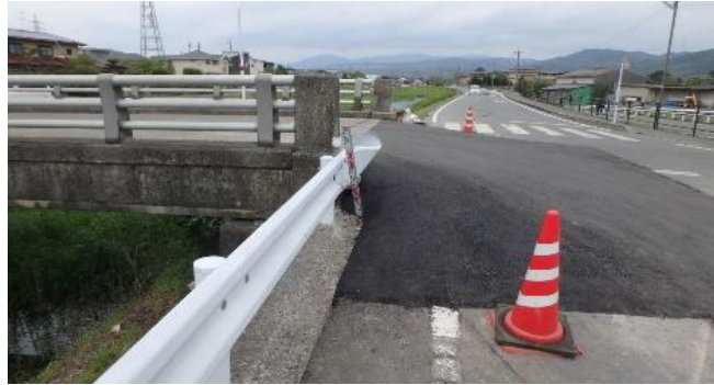
Figure 1. Ground subsidence at the back of abutment.
