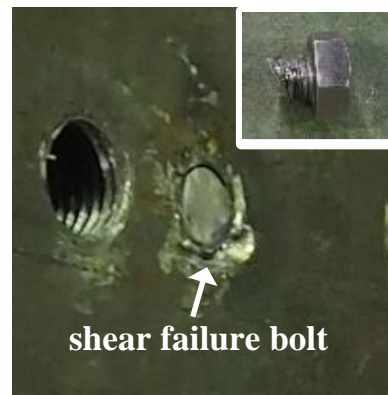
Figure 7. Shear failure bolt.
